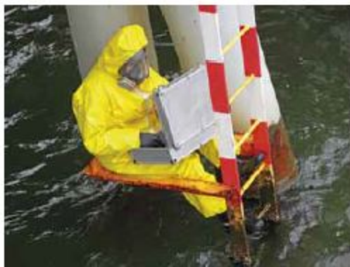
Figure 2. Suspended pipelines are difficult to inspect with manual ultrasonic methods, requiring access by boat or a ladder.
