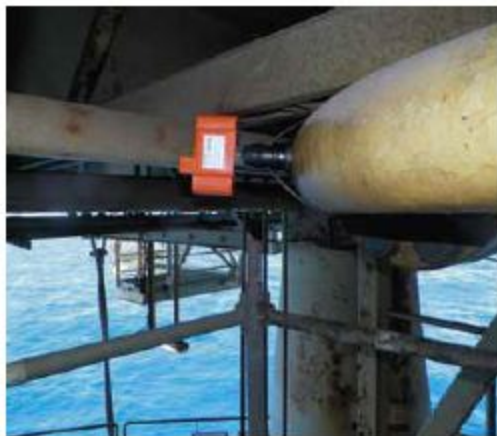
Figure 3. Permasense ET210 wireless ultrasonic wall thickness sensors provide continuous corrosion monitoring of jetty pipelines.
